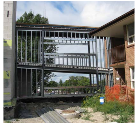
Above: Outside view of the corridor connecting the addition to the existing unit
